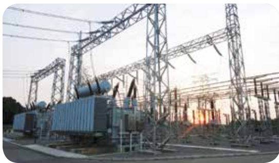
The Veyangoda 220/132 kV Grid Substation, which will be augmented under this project
